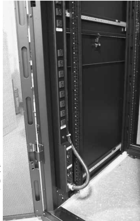
Power Commander Plus High Current Power Distribution Unit shown mounted in an IT cabinet.
