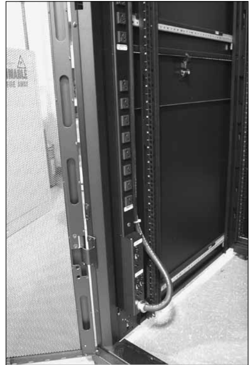
6B21N Power Commander Plus Power Distribution Unit shown mounted in an IT cabinet.
