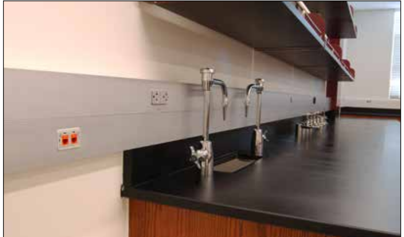
An ALA4800 Series Raceway installation in a laboratory is both functional and aesthetically pleasing.
