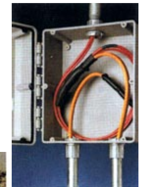
All ElectroMelt system terminations are made in the field in easily accessed junction boxes.
